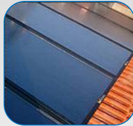
Solar heating and cooling systems
