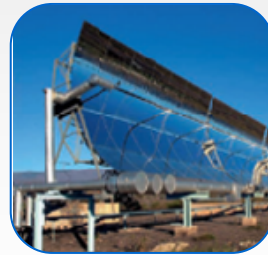
Concentrated Solar Power
