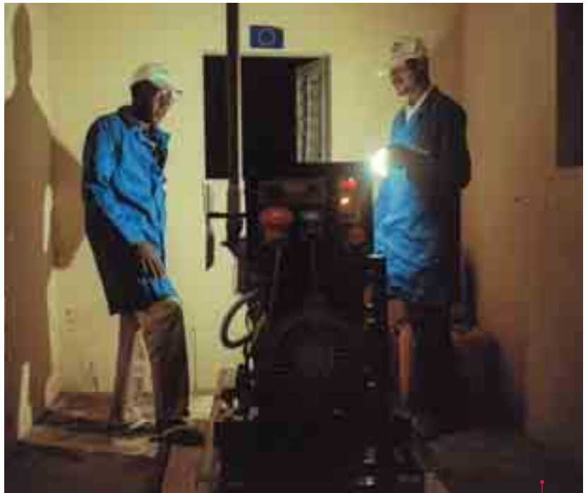
Maintenance by the local team Source: Joan Bardeletti
