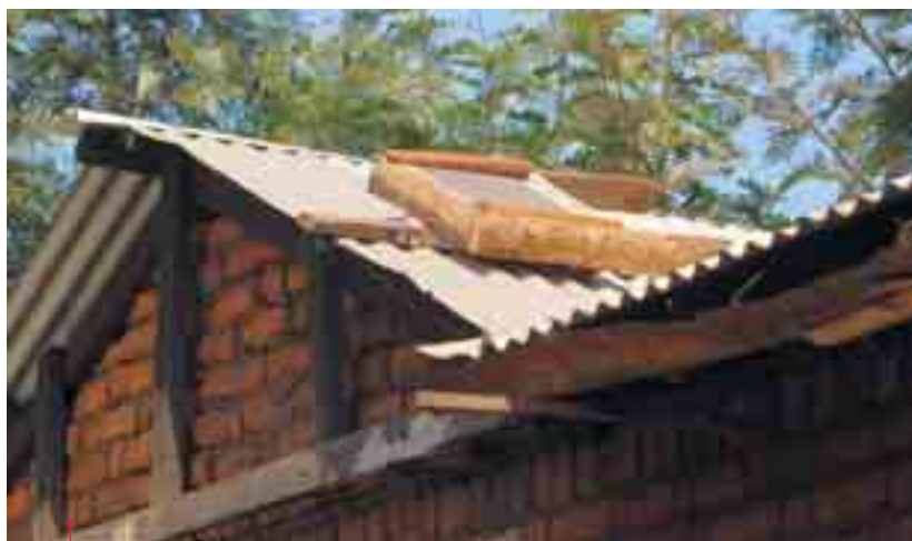
Solar panel installed on the roof of a rural house, Kenya Source: PAMIGA
