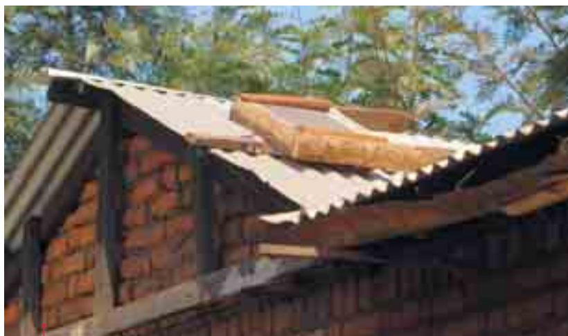
Solar panel installed on the roof of a rural house, Kenya Source: PAMIGA
